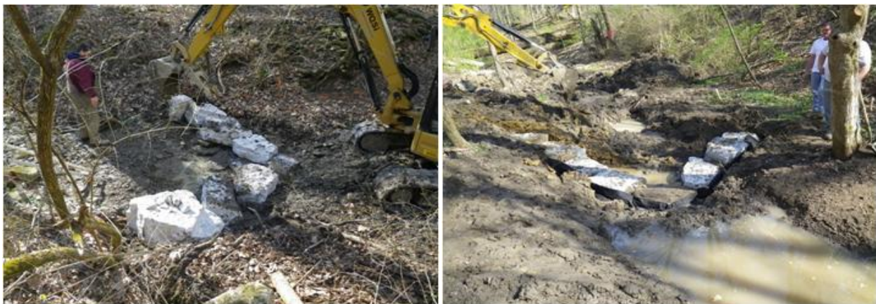
Sewer Separation, Natural Conveyance in Ault Park, Upper Duck Watershed, 2012 MSDGC. Flow previously was directed into the combined sewer; this separation project has removed an additional 100 acres of park land from draining into the combined sewer.
